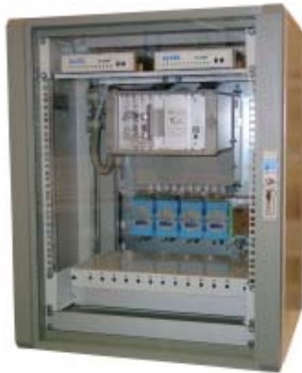
Unit with RTU-314, modems, adaptors RS485/RS232, UPS, conditioner
